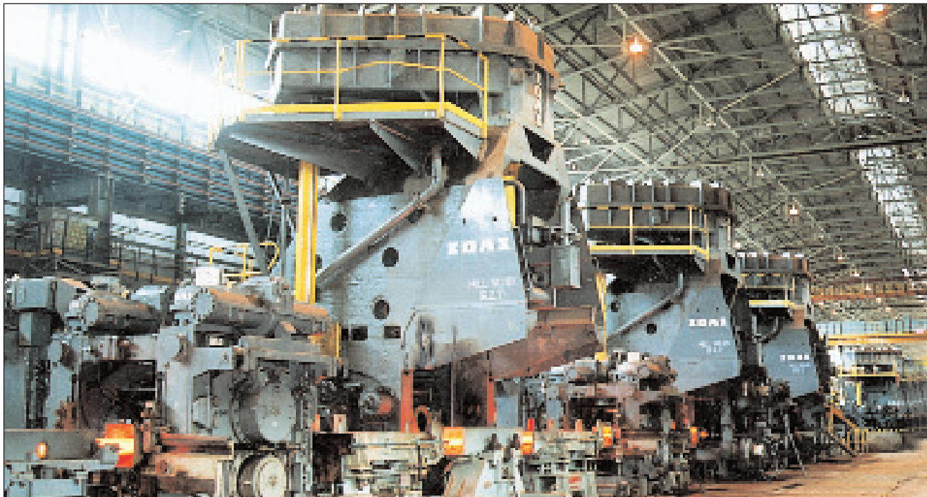
Medium Merchant & Structural Mill
